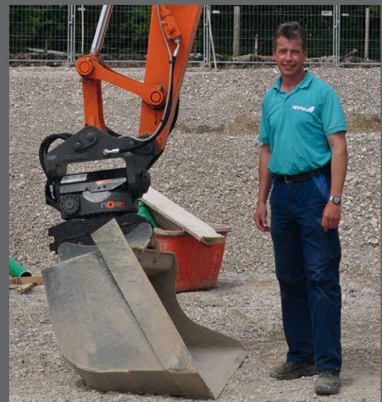
Florian Walter, operator at the company Penzenstadler, here with a TR10NOX Tiltrotator at the construction site of the OBI Hardware Store in Munich Daglfing, Germany
