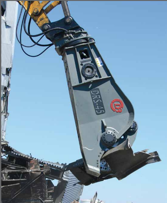
Brown & Mason at Coryton Oil Refinery
